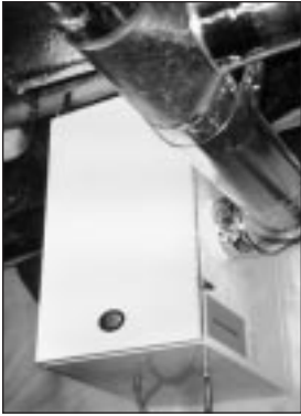
An air-to-air heat exchanger is a balanced ventilation system, meaning that it exhausts out and brings in an equal amount of air. Its heat recovery feature makes it one of the more energy efficient ventilation systems available.
